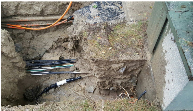
6 Figure 19: Excavated direct-buried cables near pad-mounted transformer base
